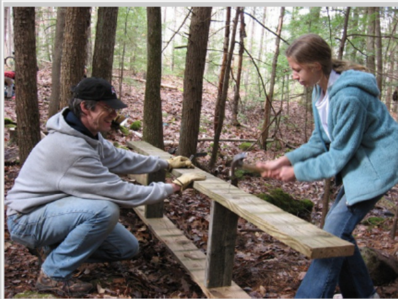
Maggie Jensen pounds nails into new bridge while her father, Jim, holds things steady
